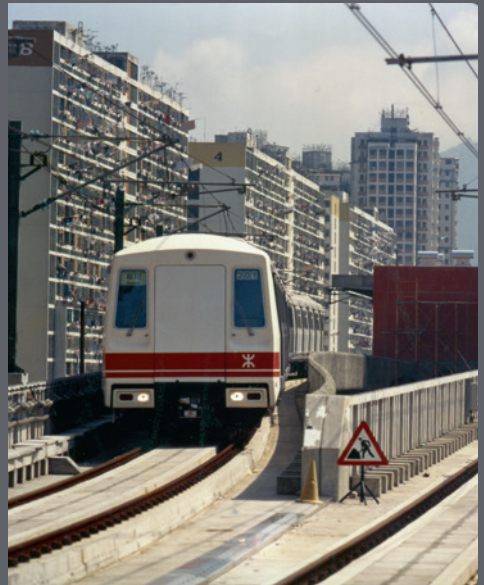
Above: Trackwork under-taken on the Hong Kong Mass Transit Railway System. Overhead section of twin track running into the partly constructed Ngau Tau Kok Station.
